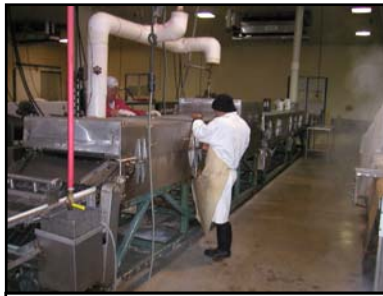
Nitrogen freeze tunnel
